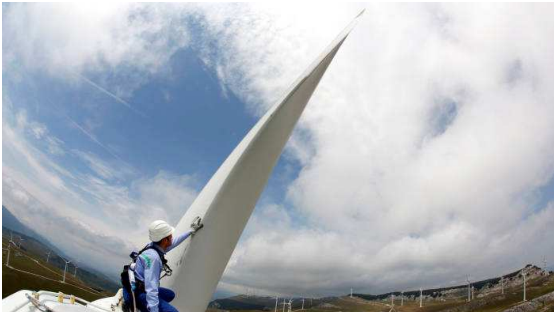
Wind Turbine Blade
